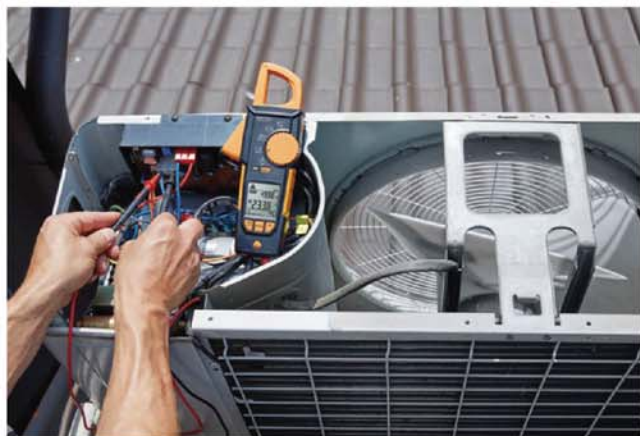
测量空调外机电压
