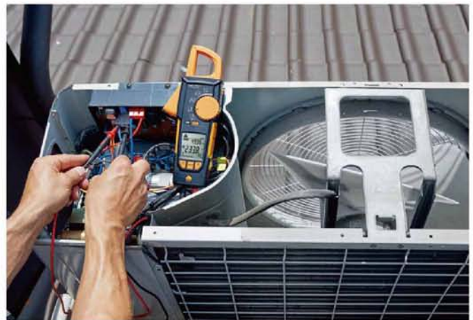
测量空调外机电压
